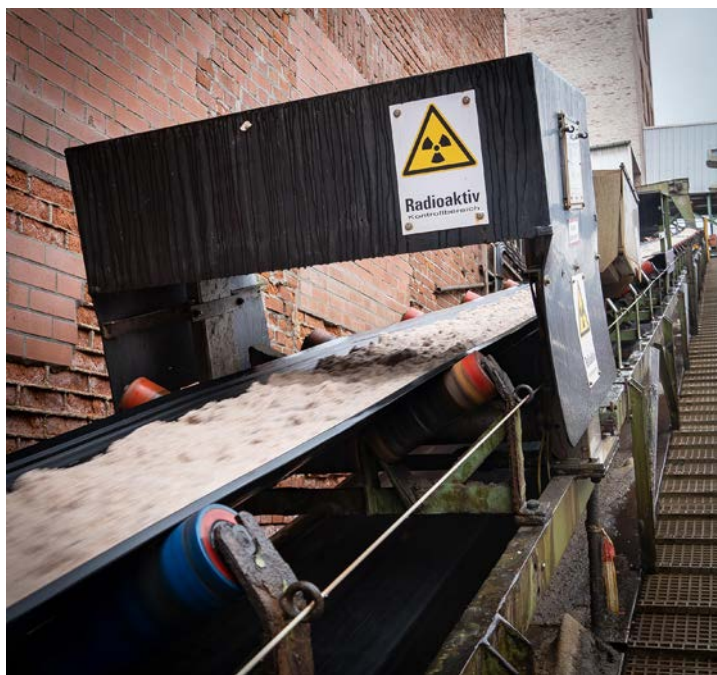
Figure 2. Radiometric bulk flow measurement system installed at an outside conveyor belt.
