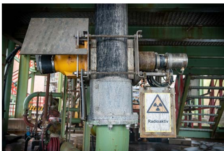
Figure 3. Radiometric density gauge installed at the outlet of a floatation tank.
